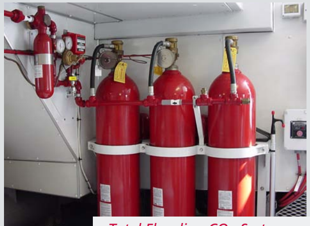
Total Flooding CO 2 System
